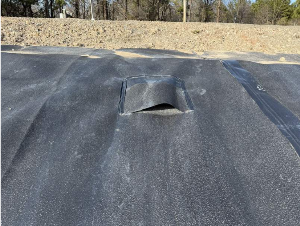
Photo 14 – Typical liner vent.
